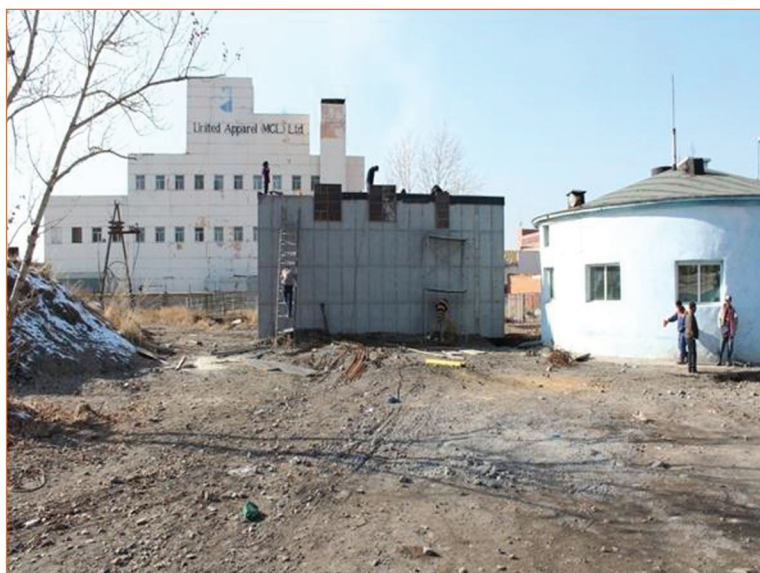
Picture 62. Expansion of the Khargia wastewater pre-treatment plant: Newly established construction with a capacity of 200-400 m 3
