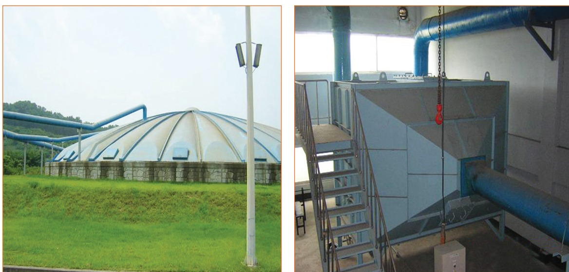
Picture 55. Sludge thickening equipment
