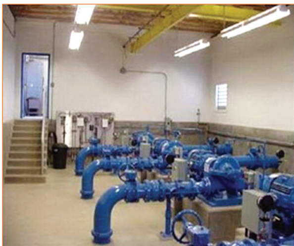
Picture 32. Pump station
