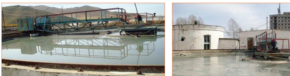
Picture 61. Khargia Industrial Wastewater Pre-Treatment Plant
