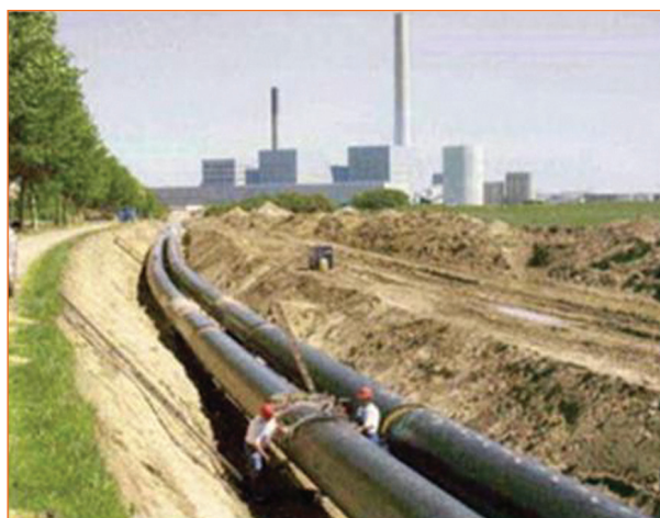
Picture 30. Pipelines used in Ulaanbaatar water supply
