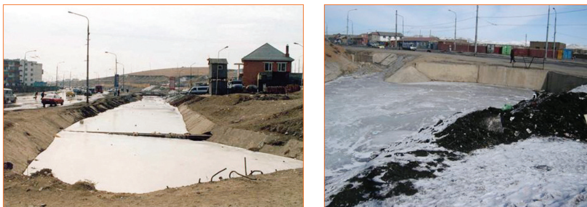
Picture 66. Appearance of flood protection channel filled with snow and ice
