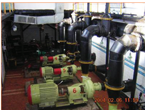
Return sludge pump
