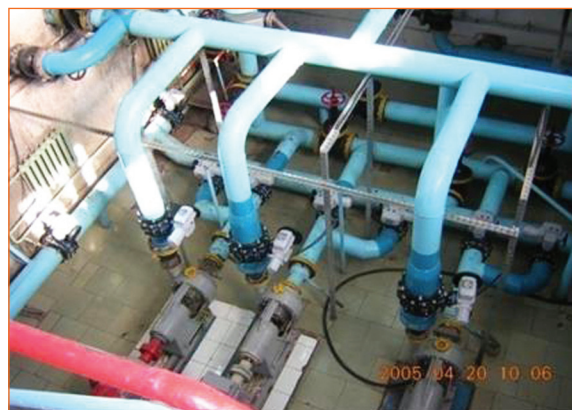
Pump station for raw residue
