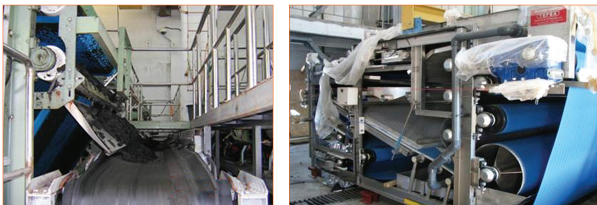
Picture 54. Sludge dehydration equipment
