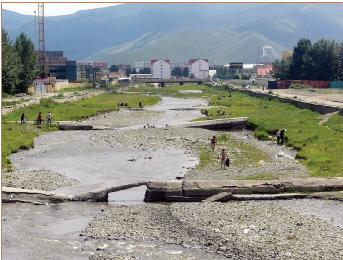
Picture 69. Flood protection channel in the Selbe River
