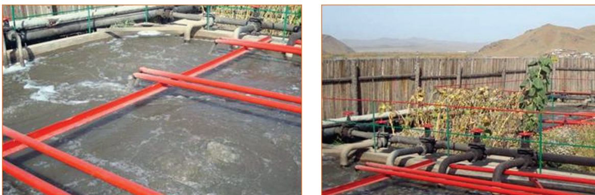
Picture 60. Bio Factory WWTP's clarifiers
