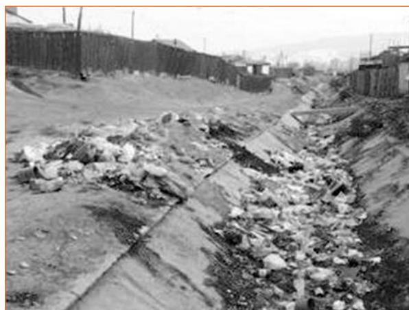
Picture 68. Wastes dumped into the flood protection channel
