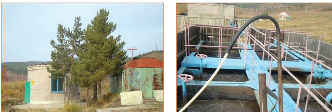
Picture 56. Bayangol WWTP
